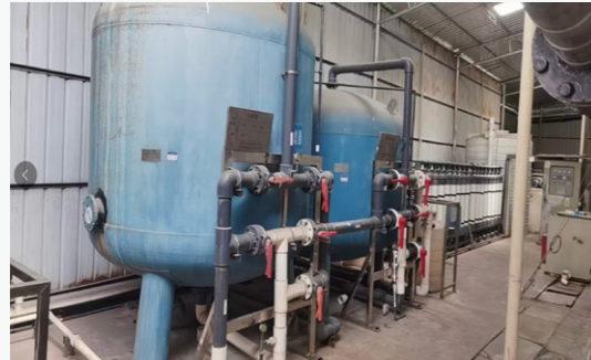
Sand Filtration Equipment
