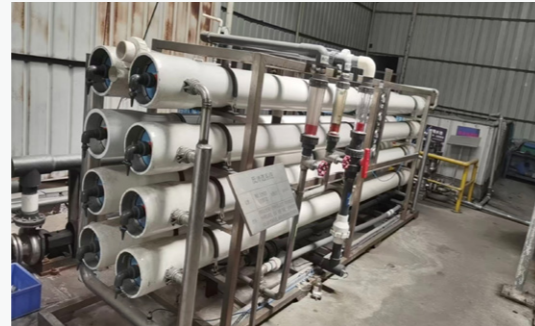
Reverse Osmosis (RO) System
