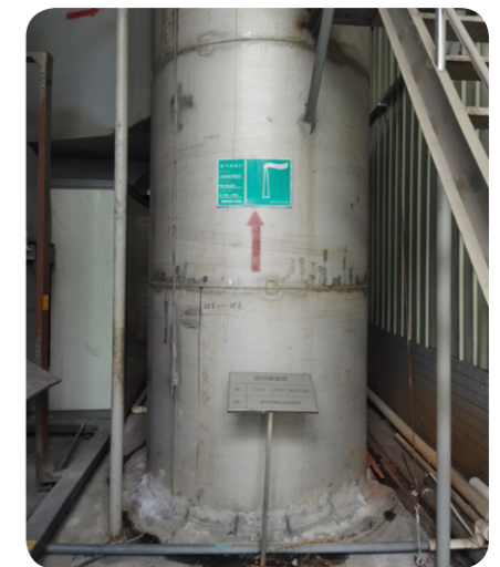
Waste Gas Treatment Facilities
